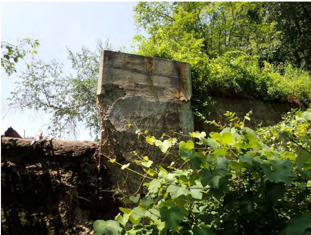
Photo 14 – Overview of downstream left wall (7/10/2019); note spalls and loose concrete materials
