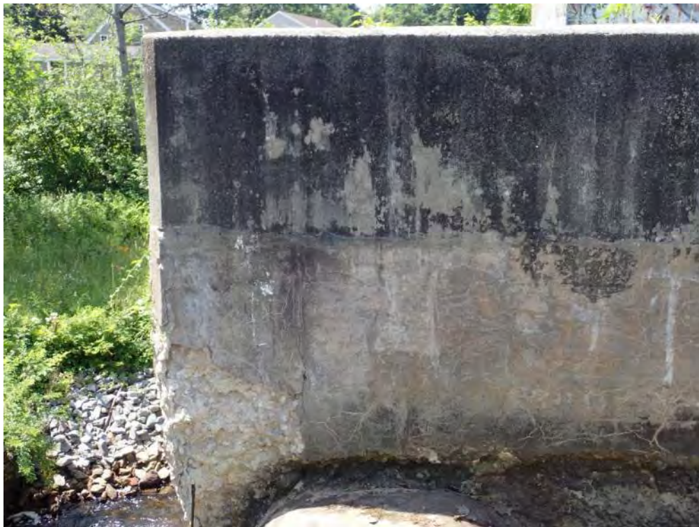
Photo 20 – Downstream side of right training wall (7/10/2019); note deterioration at waterline and large spall at downstream end
