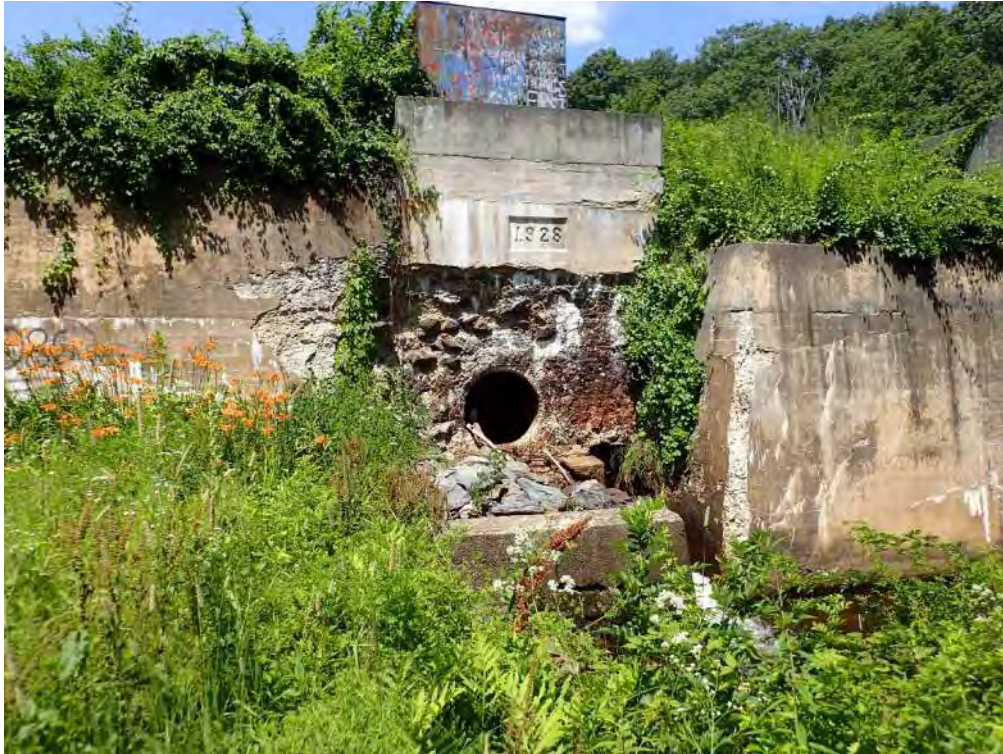
Photo 27 – Deteriorated outlet structure; note missing facing concrete (7/10/2019)
