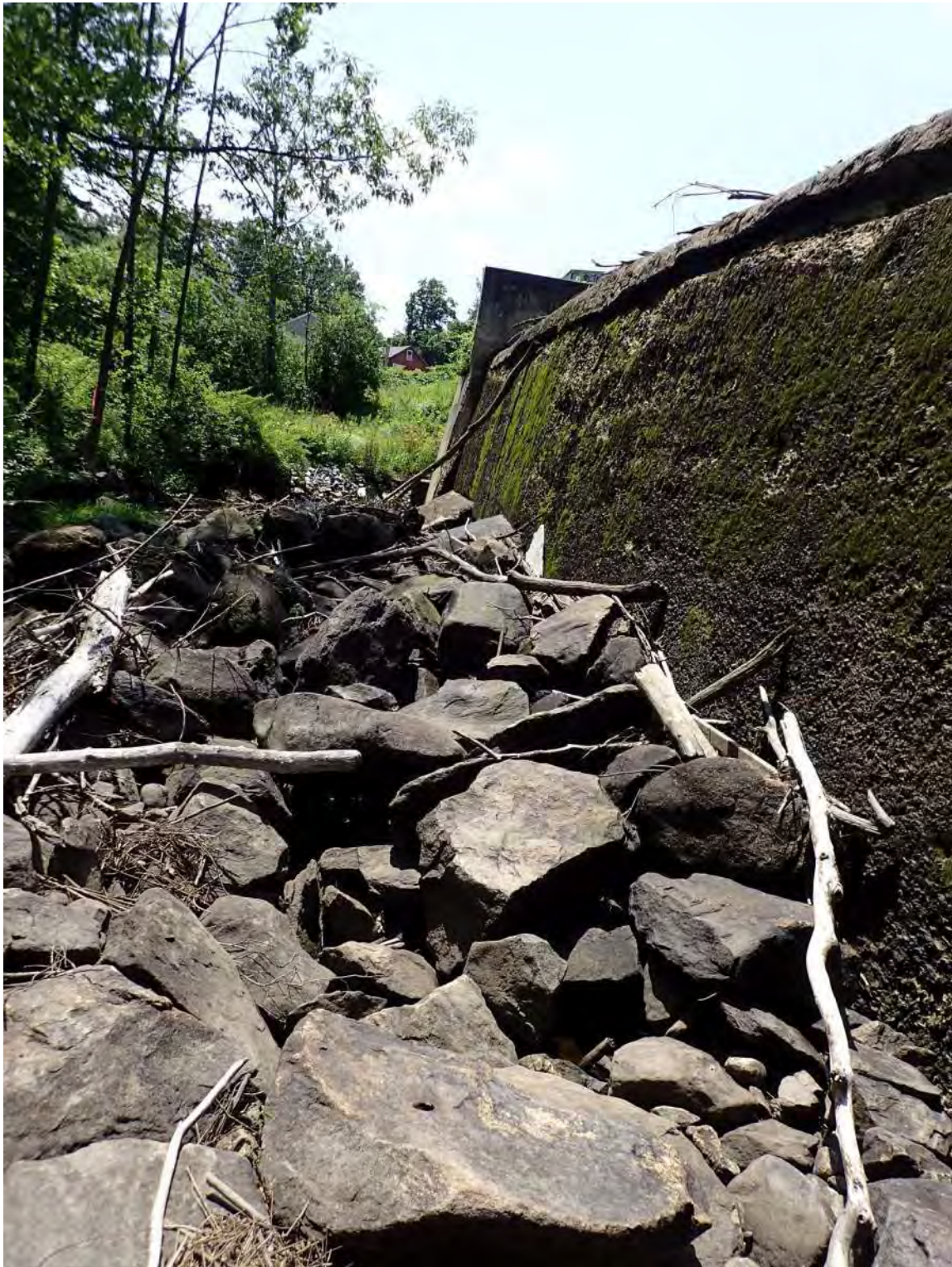
Photo 29 – Right portion of spillway looking right; note wear on face and gap at crest (7/10/2019)
