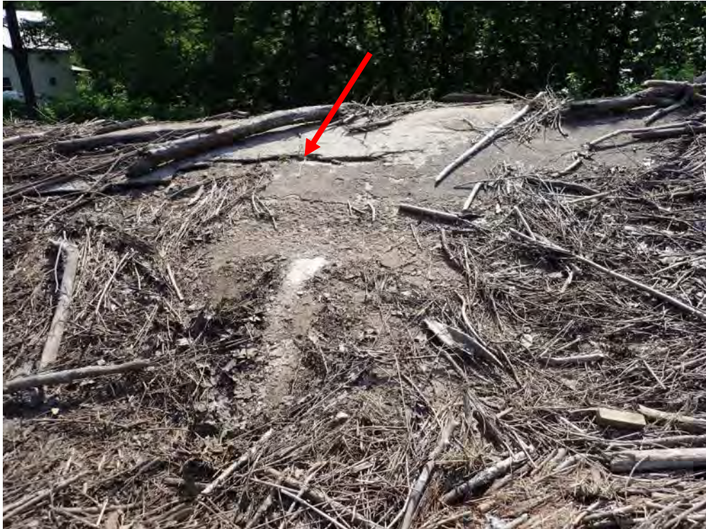
Photo 17 – View of spillway crest (7/10/2019); note separation of cap from adjacent concrete
