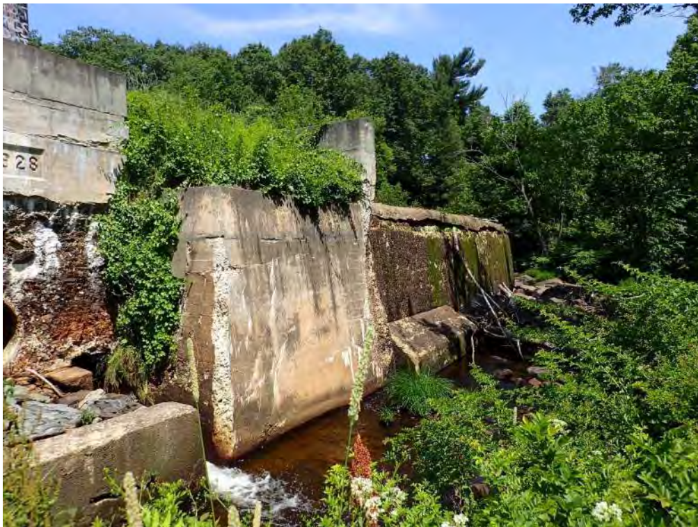
Photo 28 – Overview of downstream side of spillway at right walls; note deteriorated concrete and gap along crest (7/10/2019)
