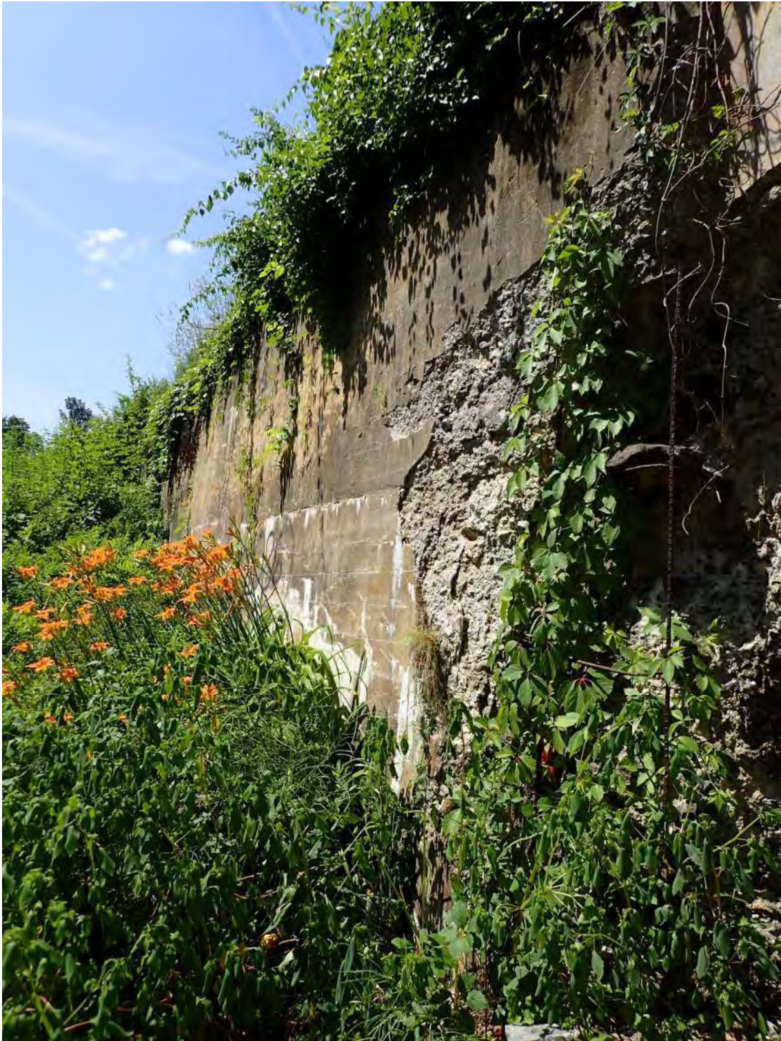
Photo 26 – Right downstream wall ; note large spall with exposed rebar (7/10/2019)
