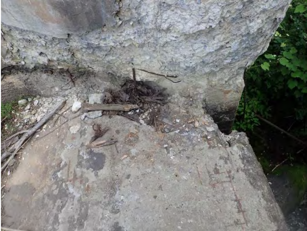
Photo 13 – Deteriorated area at left training wall – spillway interface (7/10/2018)
