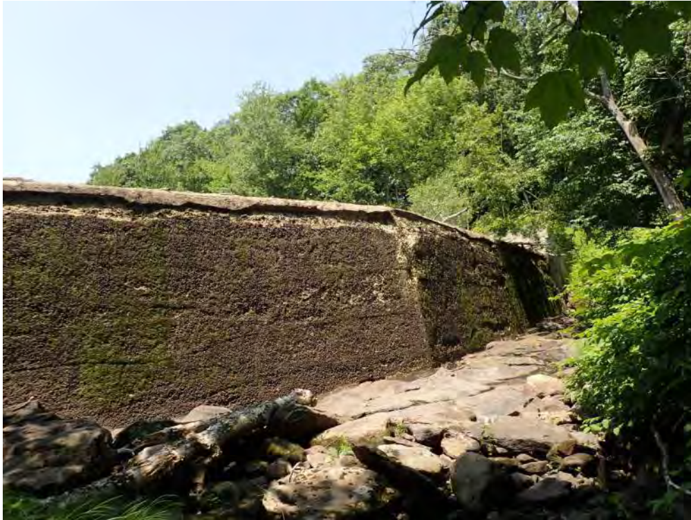
Photo 30 – Center portion of downstream face of spillway looking left; note wear on face and gap at crest (7/10/2019)
