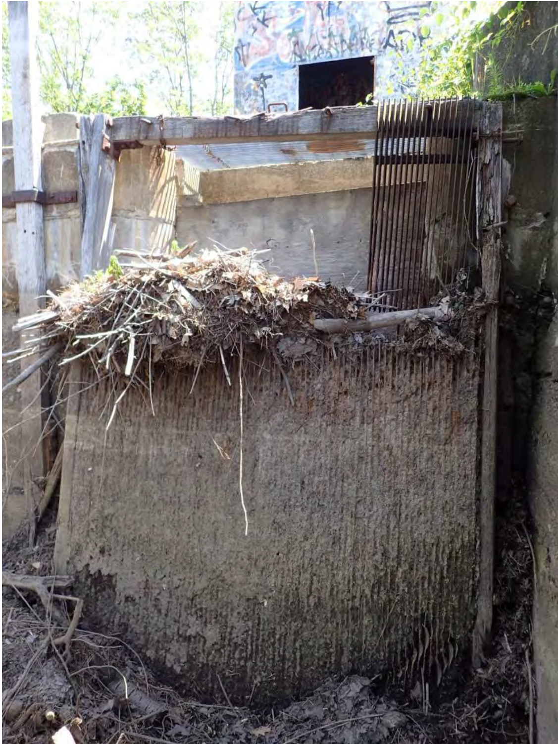
Photo 23 – Deteriorated trash racks (7/10/2019)
