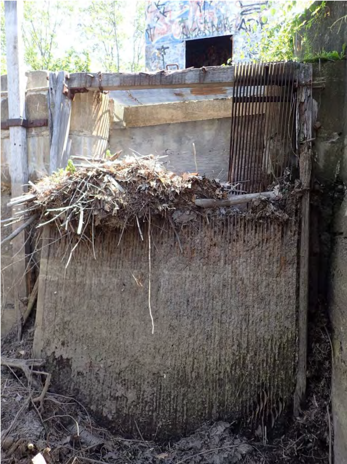
Photo 23 – Deteriorated trash racks (7/10/2019)
