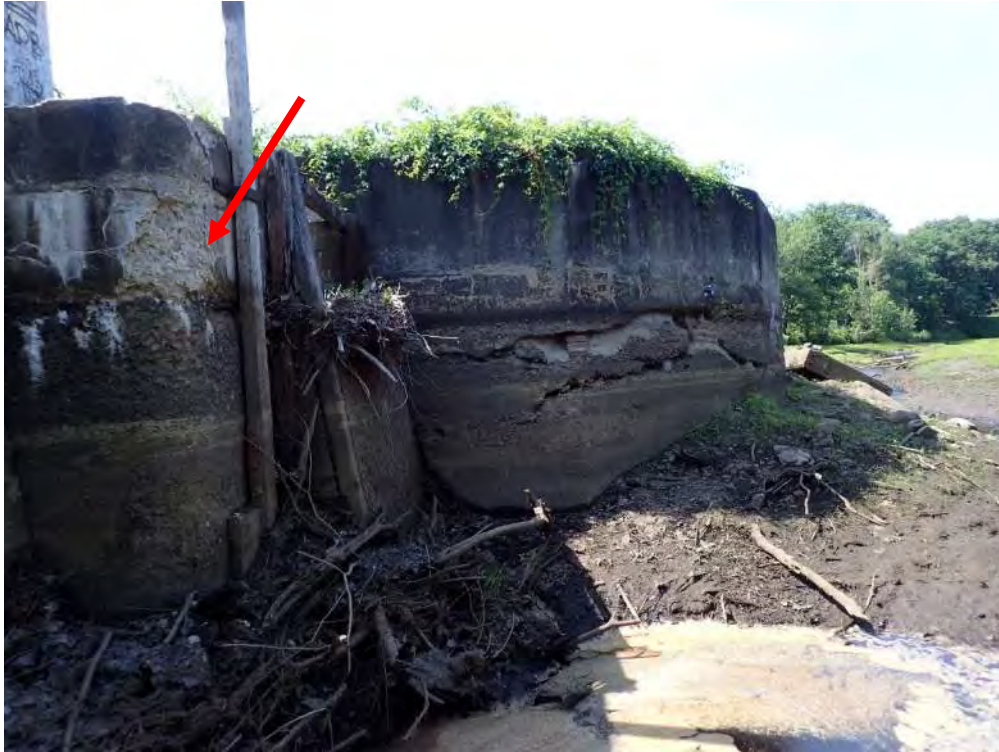
Photo 21 – Overview of outlet structure and upstream wall (7/10/2019); note irregular spalls; area of concrete breakdown indicated with arrow
