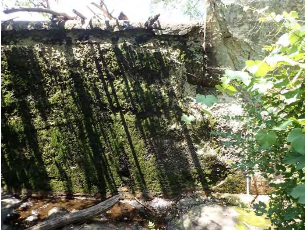
Photo 34 – Downstream face of spillway at right training wall; note large spall and heavy wear (7/10/2019)
