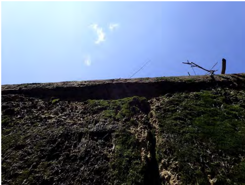
Photo 31 – Gap below crest of spillway and wear at apparent joint (7/10/2019)
