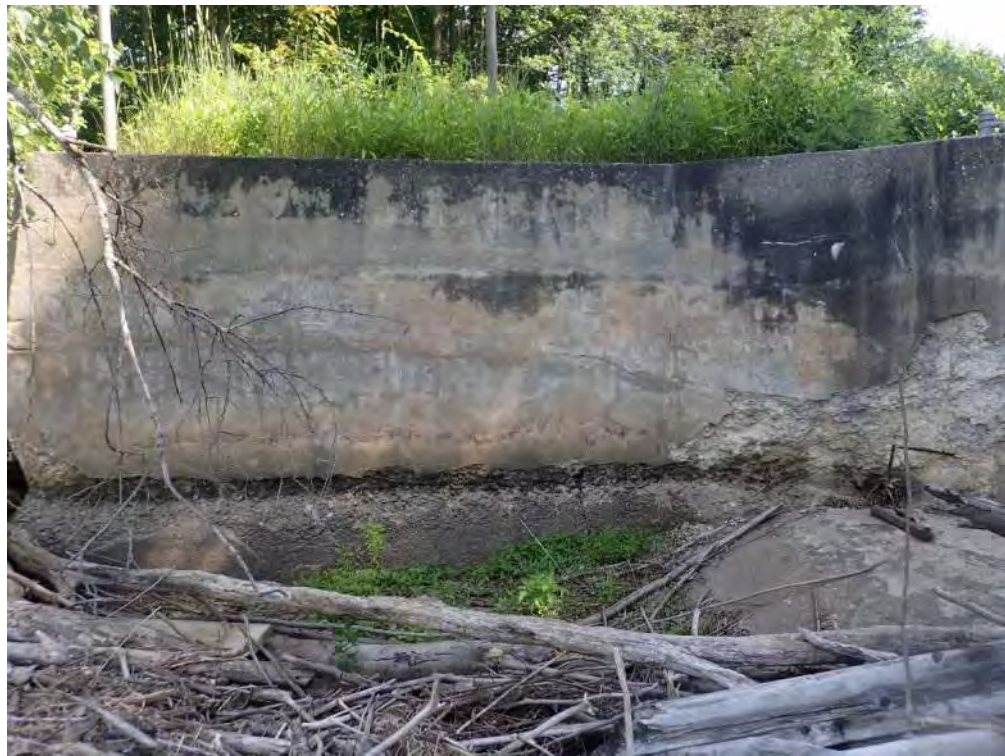
Photo 12 – Overview of left spillway training wall (7/10/2019); note deterioration along waterline
