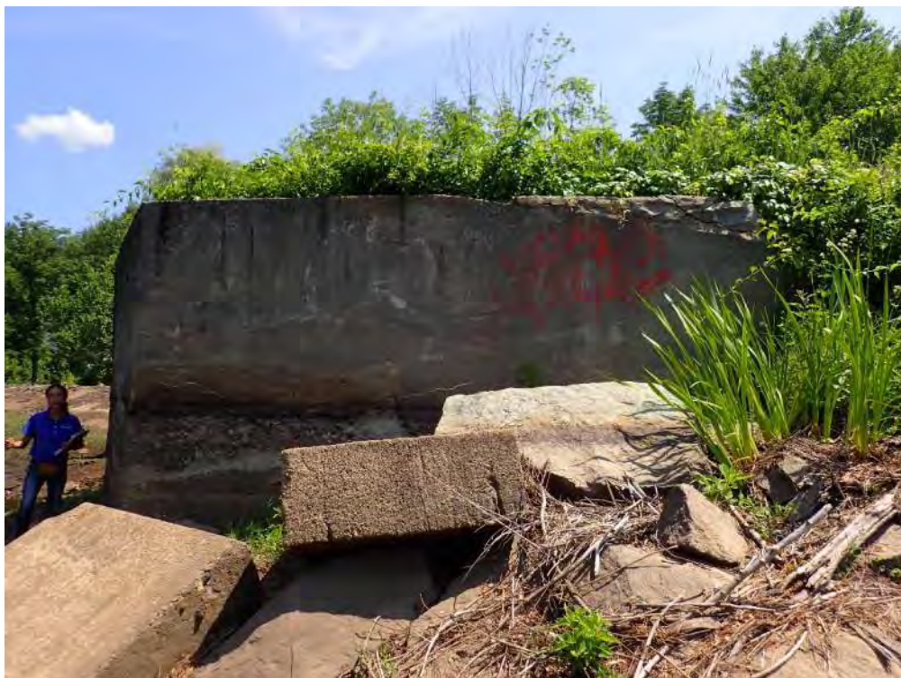
Photo 25 – Right section of right upstream wall (7/10/2019)
