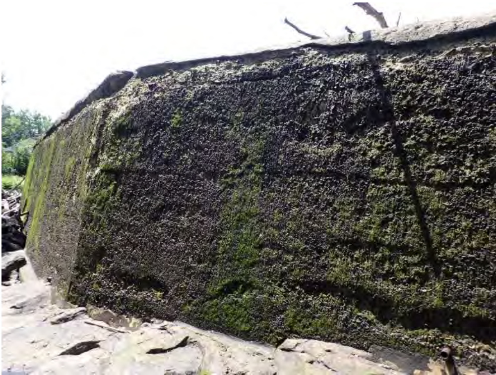
Photo 32 – Center portion of downstream face of spillway looking right; note wear on face, gap at crest, and spalls (7/10/2019)
