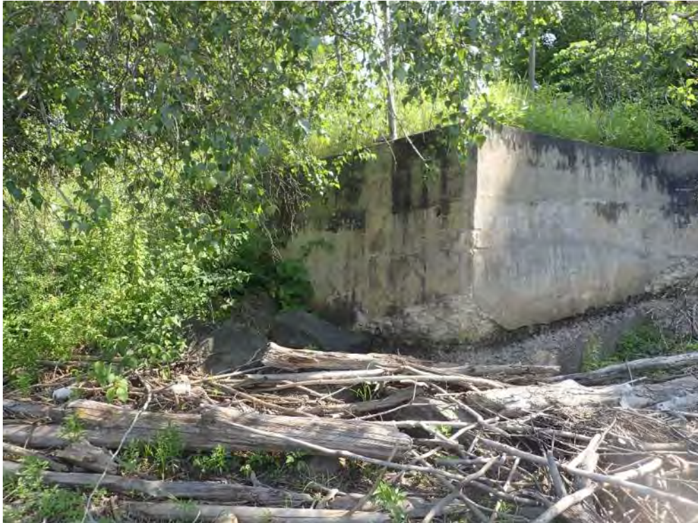
Photo 11 – Overview of left upstream concrete wall (7/10/2019); note deterioration along waterline
