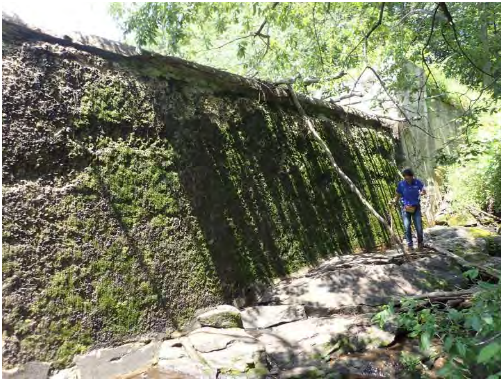
Photo 33 – Left portion of downstream face of spillway looking left; note wear on face and gap at crest (7/10/2019)
