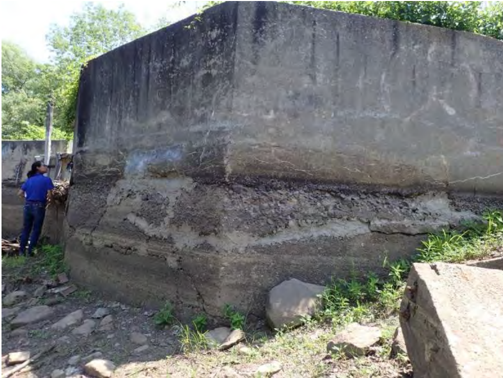
Photo 24 – Deteriorated right upstream wall (7/10/2019)
