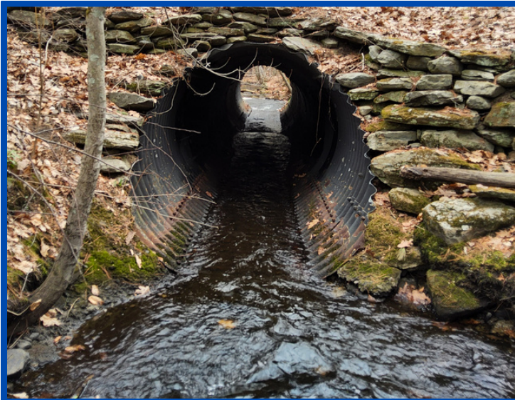
Figure 14: A round culvert that is rusted at the bottom. Stream Crossing group 2026.
