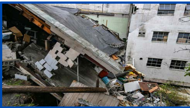
Figure 12: Collapsed building after the 2023 Leominster floods. Courtesy of Wendy Wiiks.
