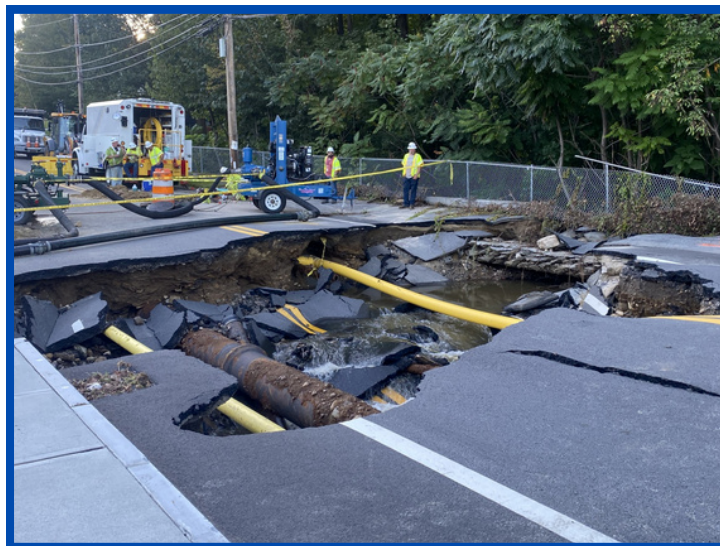
Figure 3: Leominster MA road washout at stream crossing as a result of 2023 flooding (Wendy Wiiks 2023)
