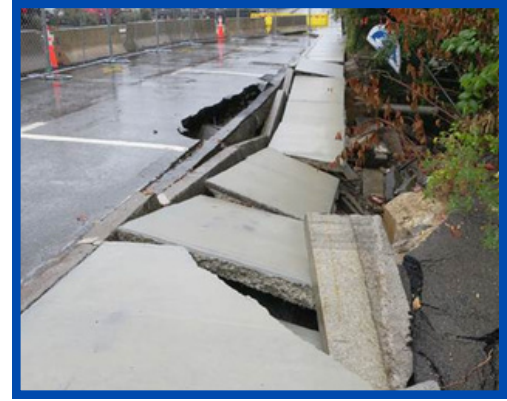
Figure 13: A collapsed road and sidewalk after the Leominster 2023 floods. Courtesy of Wendy Wiiks.
