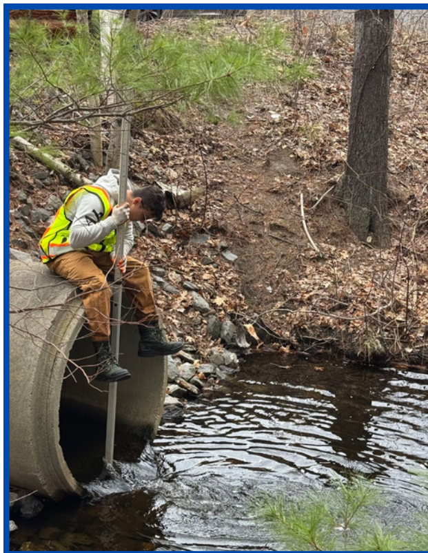
Figure 4: Five foot concrete pipe culvert with outlet drop and scour pool
